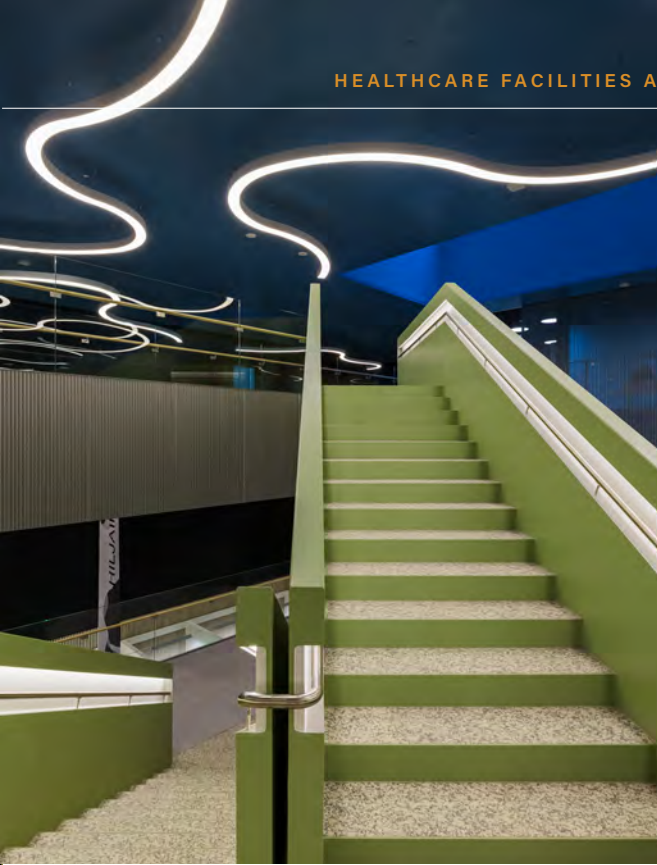
Hospital Nova is installed with the latest Helvar Insights to support a people-centric service and understanding how their facilities are used.
